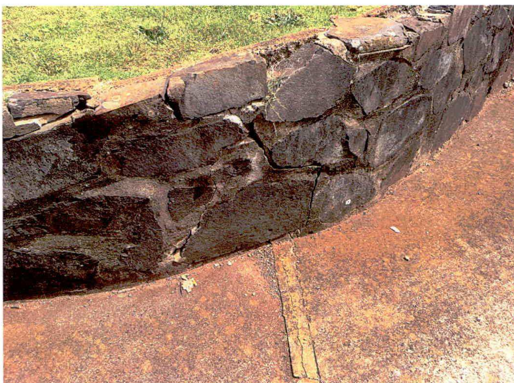
Figure 3 – Damaged section of retaining wall
