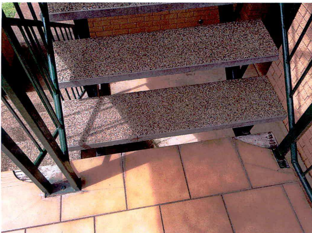
Figure 3 – Damaged landing tiles
